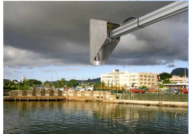
GLOSS sea level stations employ a number of instruments to measure sea level, including down-looking radars to measure sea level. Port Louis, Mauritius. Photo courtesy of University of Hawaii Sea Level Center.
