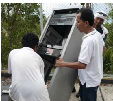
Technicians are setting up a repeater unit on Argopeni Hill in Kebumen
